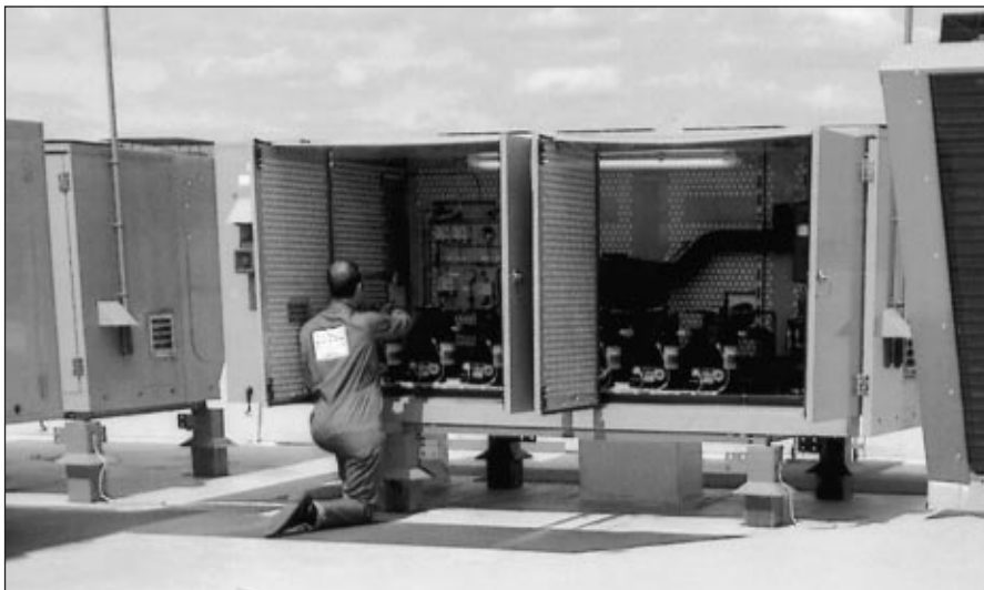
Figure 31 A roof-top hydrocarbon chiller
